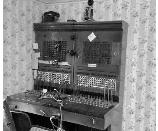
One of Lima's earliest switchboards. It is one of only two of its age surviving in New York State, thanks to the efforts of Harold Hennessey who had it donated to the Lima Historical Society. Come see it in person.
